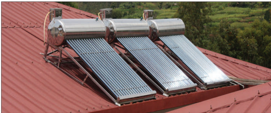
Figure 6.13: In Rusizi, solar heating panels on a roof of a house
